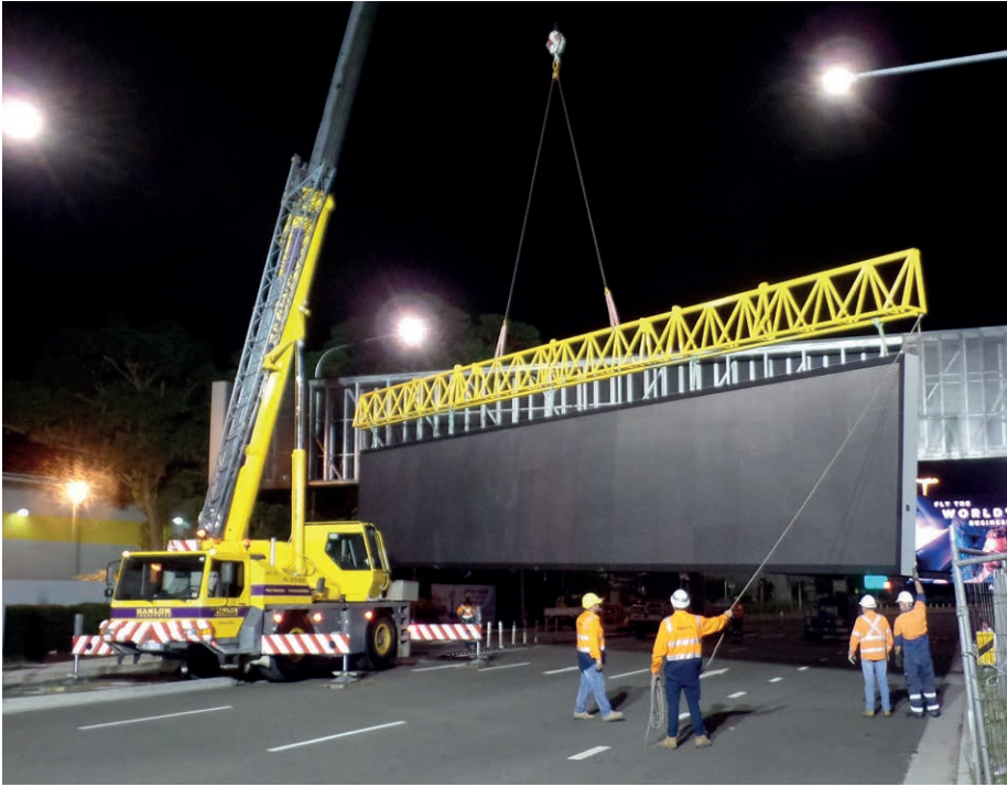
The installation took only a few minutes with little downtime for traffic
